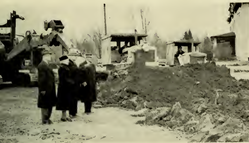
steam shovel prepares ground for new Bethel Home, Ossinger, N. Y., as (from left) Leslie J. Tompkins, Mrs. Alma Pearson, the Rev. Daniel D. Brox, executive director, and August Rosengren inspect work. The present structure (right) will be demolished.
